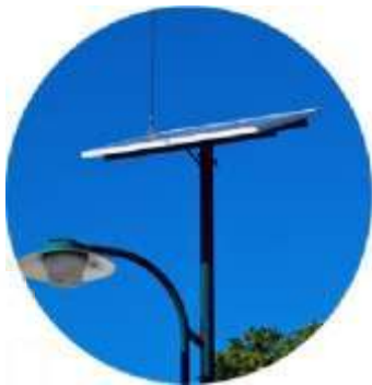
Solar Street Lights
